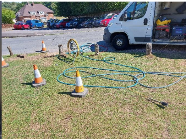
Camera where pipes are out of line
